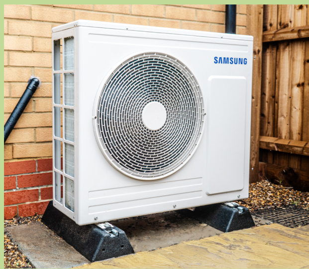
Airsource heat pump installation.
